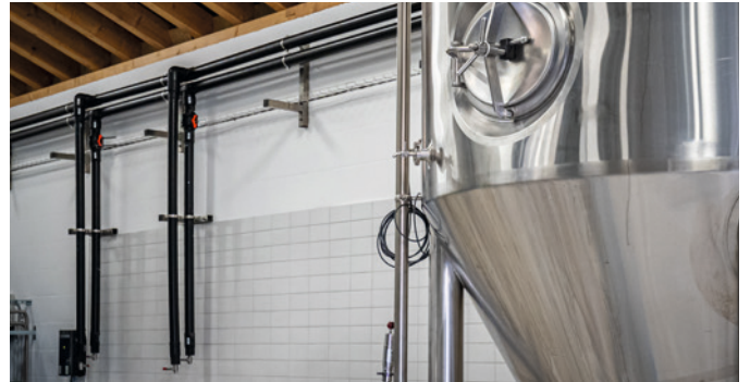
The two master brewers were able to cut the already pre-insulated plastic pipes and install them in a single session as desired without any previous expertise.
