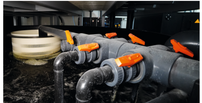
Water values always under control: industrial skimmer and denitrification.
